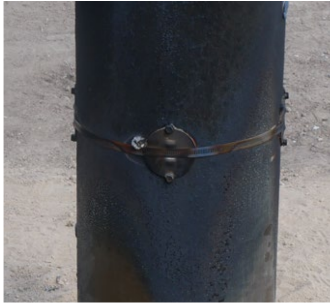
Post Fire Inspection Irreversible Temperature Measuring Device Access Cover Plate.
