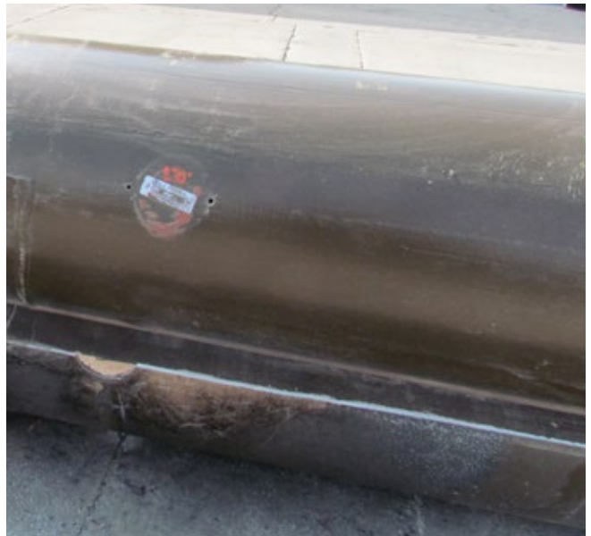
The uncompromised FRP pole after the charred outer sleeve has been removed post-fire.
